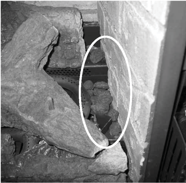
Right side of Burner
