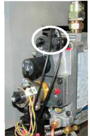
DC Sparker Wires
