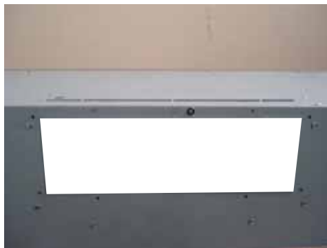
Horizontal Ducting (3-1/4"x10" Rectangular)
