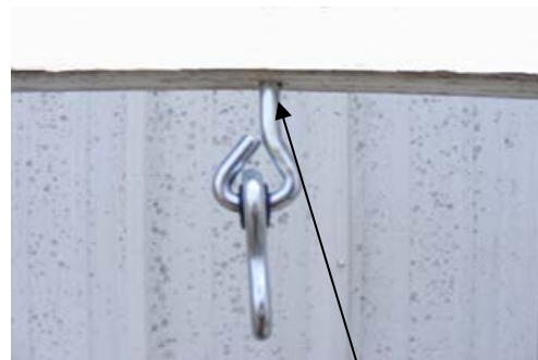
CORRECT NO EXPOSED THREADS
