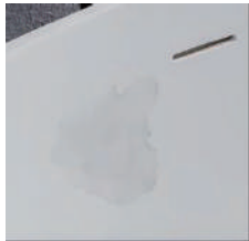
Water Stains/Light Stains
