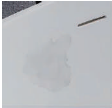
Water Stains/Light Stains
