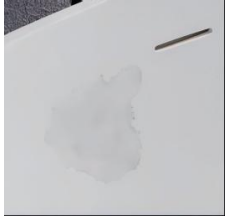
Water Stains/Light Stains
