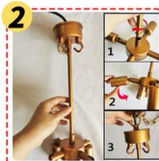
Install the lamp body according to above steps.
