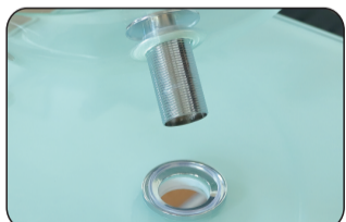
Align the sink with the drain hole and set it up (Thread seal tape five or six laps)
