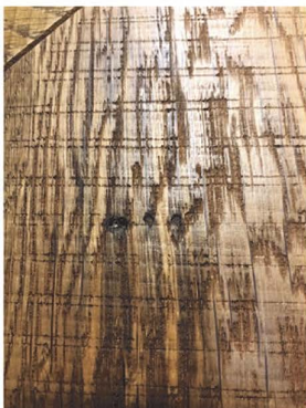
PIN/ WORM HOLES & SAW MARKS
