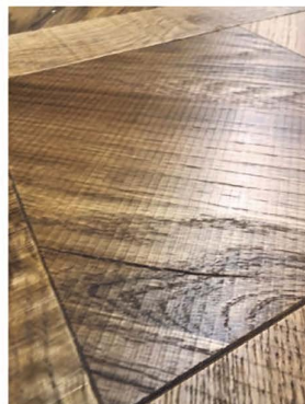
SPLITS IN TIMBER/ SAW MARKINGS
