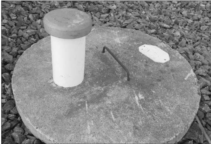
Septic tank with a vent pipe that may need to be shortened.
