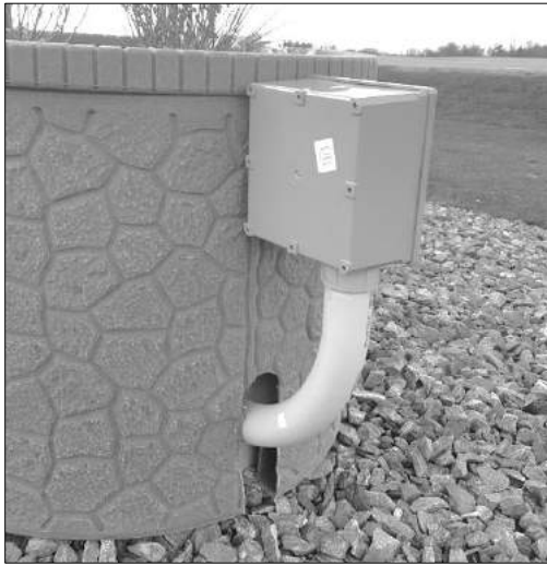
Septic tank with an electrical conduit.
