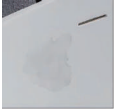
Water Stains/Light Stains
