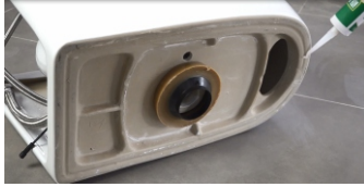
10. Apply some glass glue on the bottom of the toilet (The glass adhesive in the picture needs to be purchased by oneself.)
