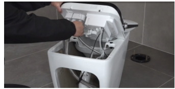
8. Take off the whole toilet seat and unscrew the flexible tube and black wire
