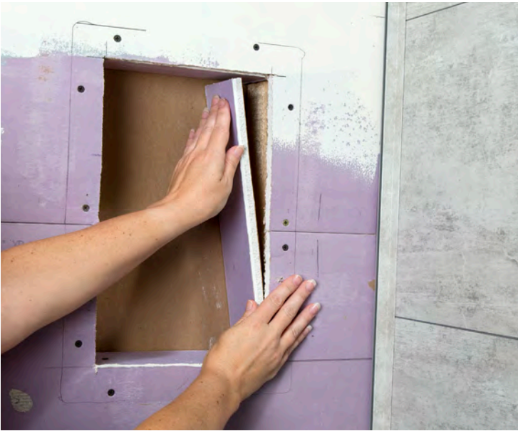
Line framed structure with waterproof board and seal joints with sealant, ensuring a waterproof seal.
