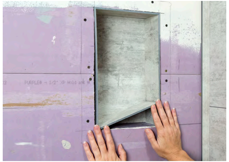
Cut sections of Paliade to line the inside of the niche. Measure and cut Paliade tiles so that they terminate at the niche opening. Apply a generous amount of the approved adhesive to the rear of the Paliade tiles to ensure proper adhesion over the ledge of the niche (where it transitions from the water board to the niche). Adhere tile pieces to the inside of the niche.
