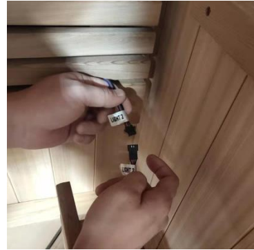
Rear Right – Corner Light Connection
