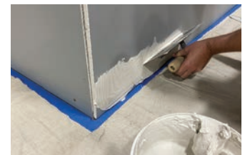
Even out adhesive with the tooth side of the trowel after it has been applied.
