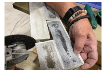
Shown here is a detail of trimming the last piece to fit into the outside corner piece that will be on the right end of the row.
