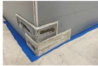
If using an outside corner piece in your design, make sure you dry fit it first and the grout edge is on top.
