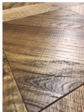
SPLITS IN TIMBER/ SAW MARKINGS
