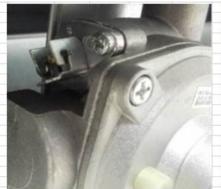
Fig. 11a: Open shut-off valve
