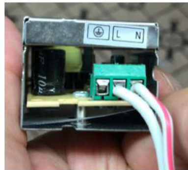
Figure 3 - Cables attached to power supply unit
