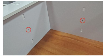
9. THERE ARE HOLES AT THE JOINTS OF EACH PLATE
