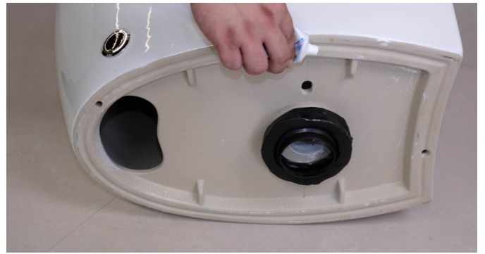
12. Apply a layer of silicone sealant to the base of the toilet. ( The silicone sealant adhesive in the picture needs to be purchased by oneself. )
