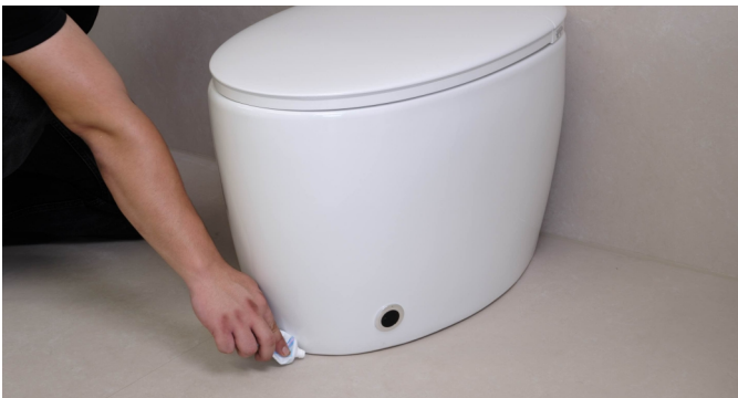
18. Apply some silicone sealant to fix the toilet and insulate the outside dirt from entering. ( The silicone sealant adhesive in the picture needs to be purchased by oneself. )
