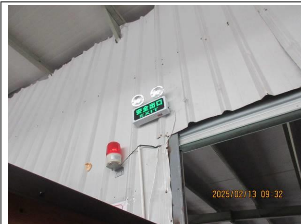
Emergency exit sign, fire alarm and emergency lighting
