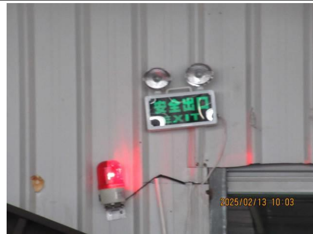
Fire alarm test
