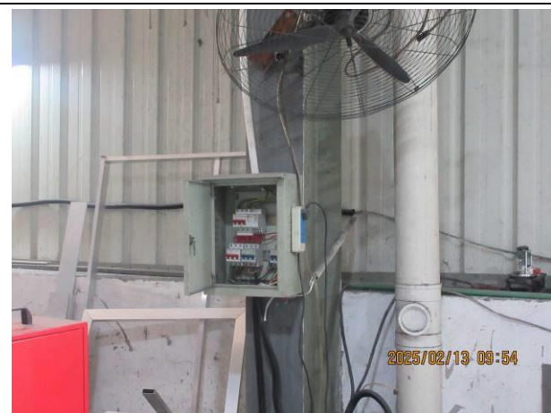
NC: Electrical box was not locked
