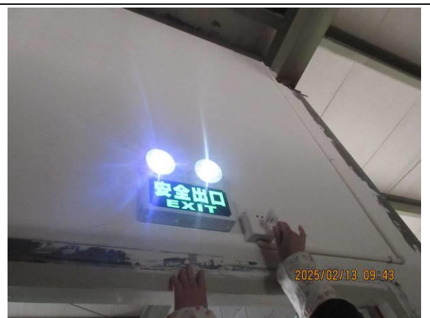
Emergency lighting test
