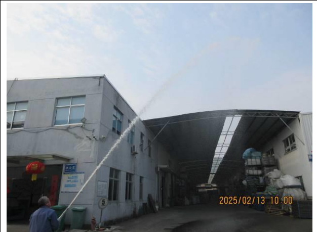
Fire hydrant test
