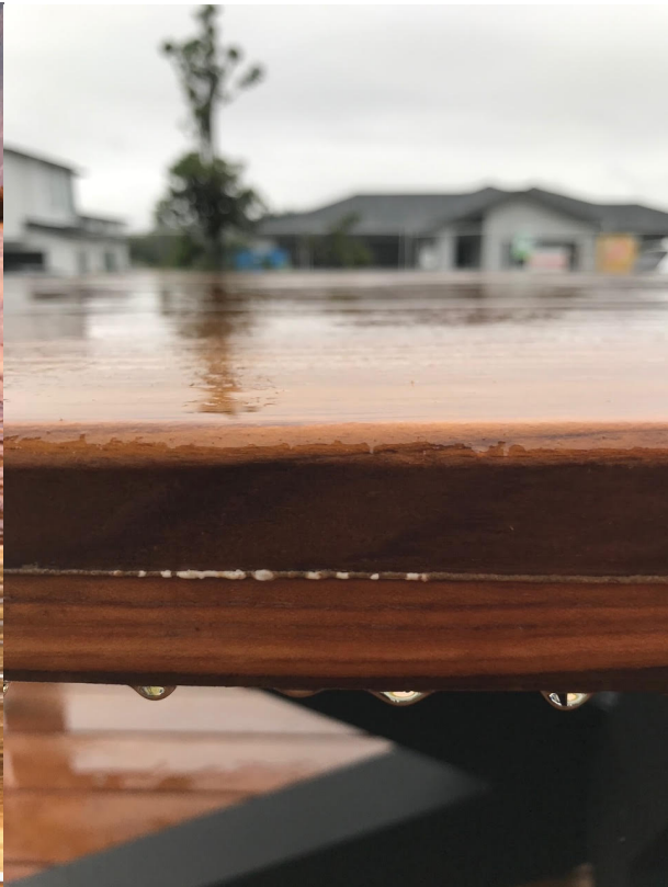
GLUE LINE AT LAMINATION
