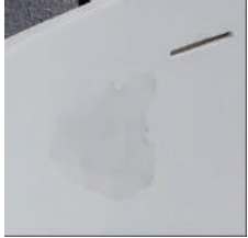
Water Stains/Light Stains
