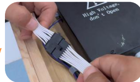
Wires of control panel
