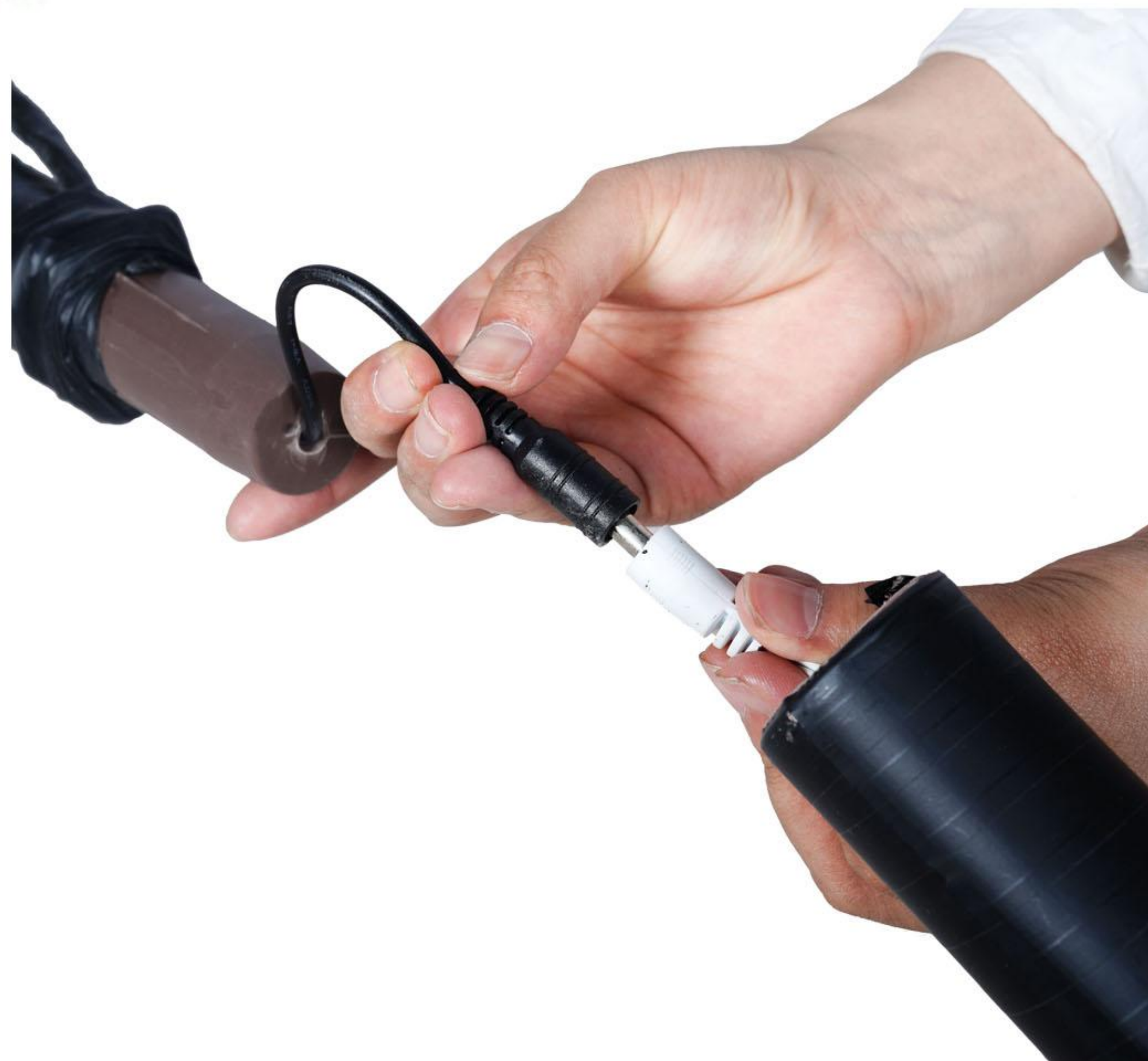
Connect the wire inside section A and B
