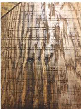
PIN/ WORM HOLES & SAW MARKS
