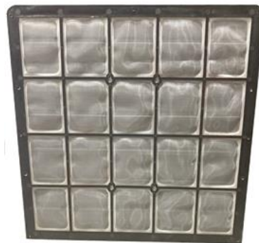
Screen removed from access door
