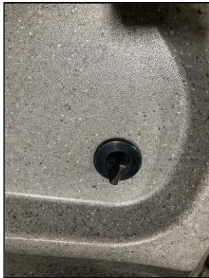
The air bleed valve closed.
