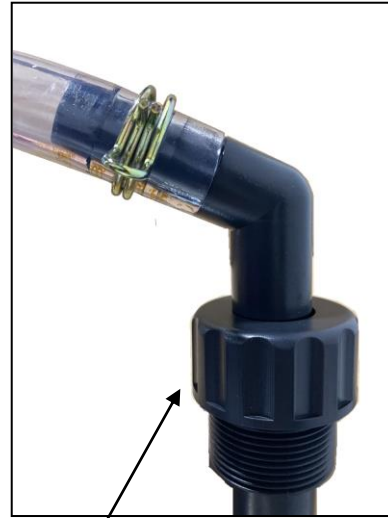
The chiller union.
