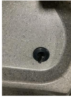
Air bleed valve closed
